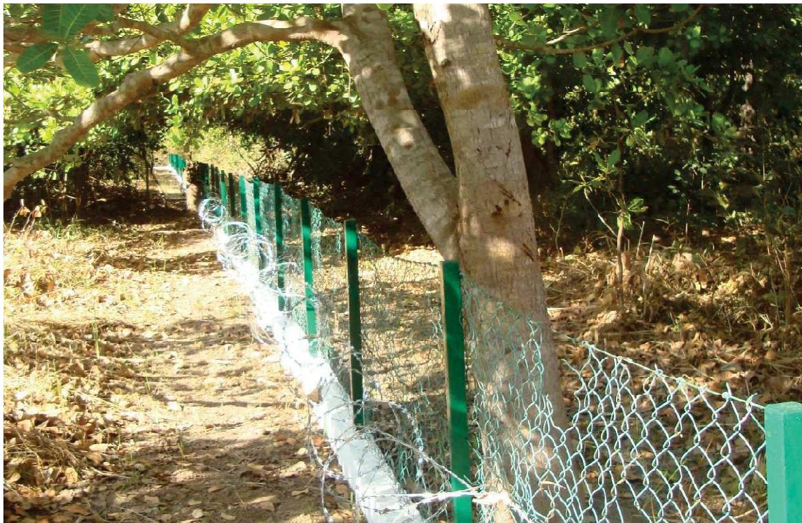
Repaired fence to keep the many goats of the village, that have in the past caused enormous damage to the huts, and to the vegetable and the botanical garden around Casa Daridibó, out of the camp site
